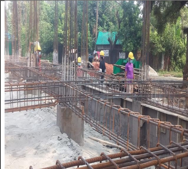
Construction work of Akrul Govt. Primary School through PEDP-4 under LGED, Upazila: Keranigonj, District: Dhaka|
