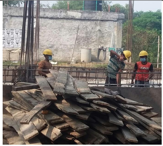
Construction work of Bir Baghoir Govt. Primary School through PEDP-4 under LGED, Upazila: Keranigonj, District: Dhaka
